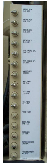
MAIN FRAME BANK 2
